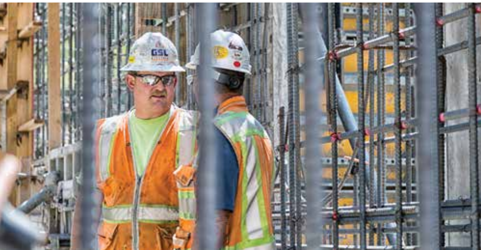
Employee-owners at GSL Electric, like Project Superintendent Wade Remington, shown here, work closely with clients on key points, such as this schedule review with the general contractor of a project in downtown Salt Lake City.
