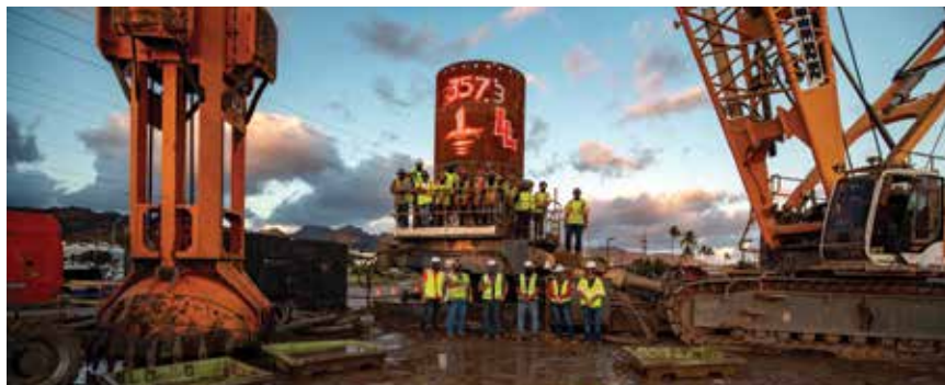
This team of experts solved major access and geological issues to ensure successful installation of the world's largest and deepest oscillated shaft for the Honolulu Authority Rapid Transportation project between Aloha Stadium and Middle Street in Honolulu.
